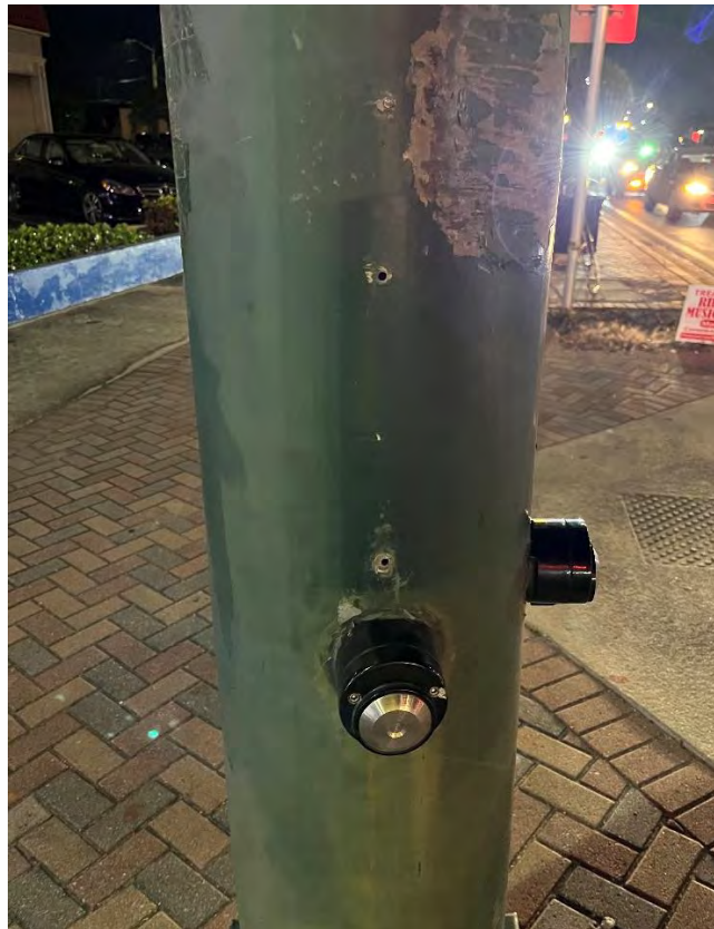
Exhibit 33: Missing Pedestrian Traffic Signal (Walk/Don't Walk) Signs
