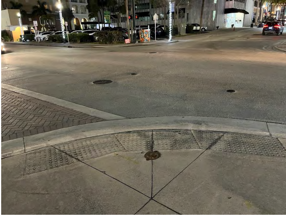
Exhibit 32: Missing ADA Compliant Sidewalk
